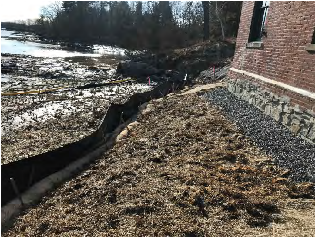
Fig 2: Slope between the cable house and salt marsh restoration at the Eversource property/west side of the bay. Viewing south. (01-19-21)
