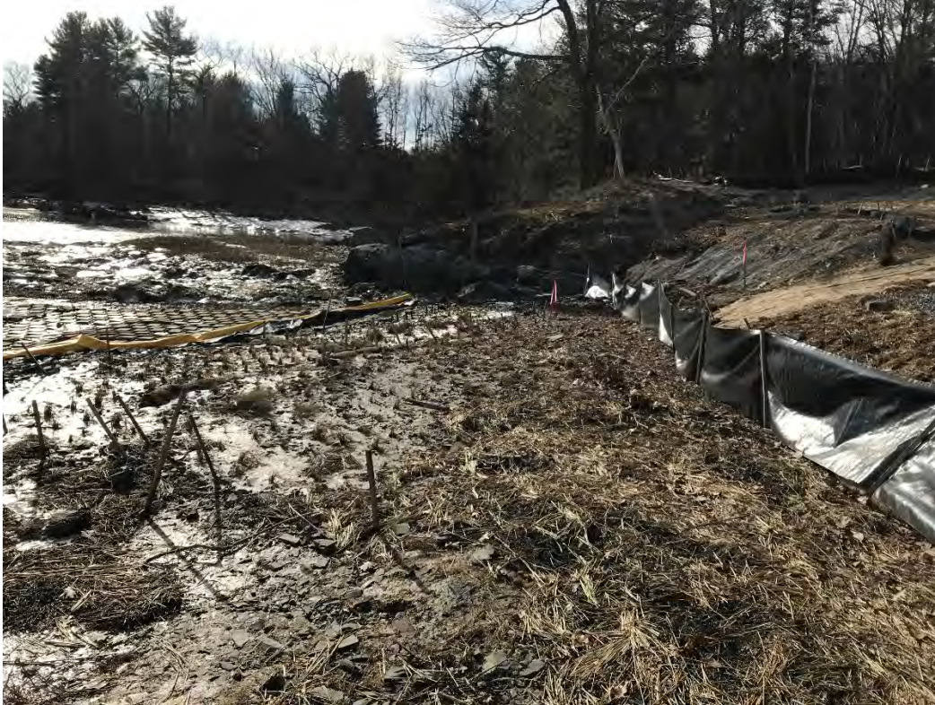
Fig 3: Toe of the slope and salt marsh restoration at the Eversource property/west side of the bay. Viewing south. (01-19-21)
