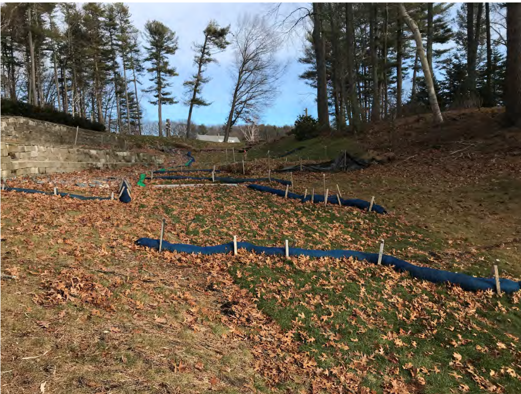
Fig 9: Slope below the manhole at Gundalow Landing/east side of the bay. Viewing east. (01-16-21)
